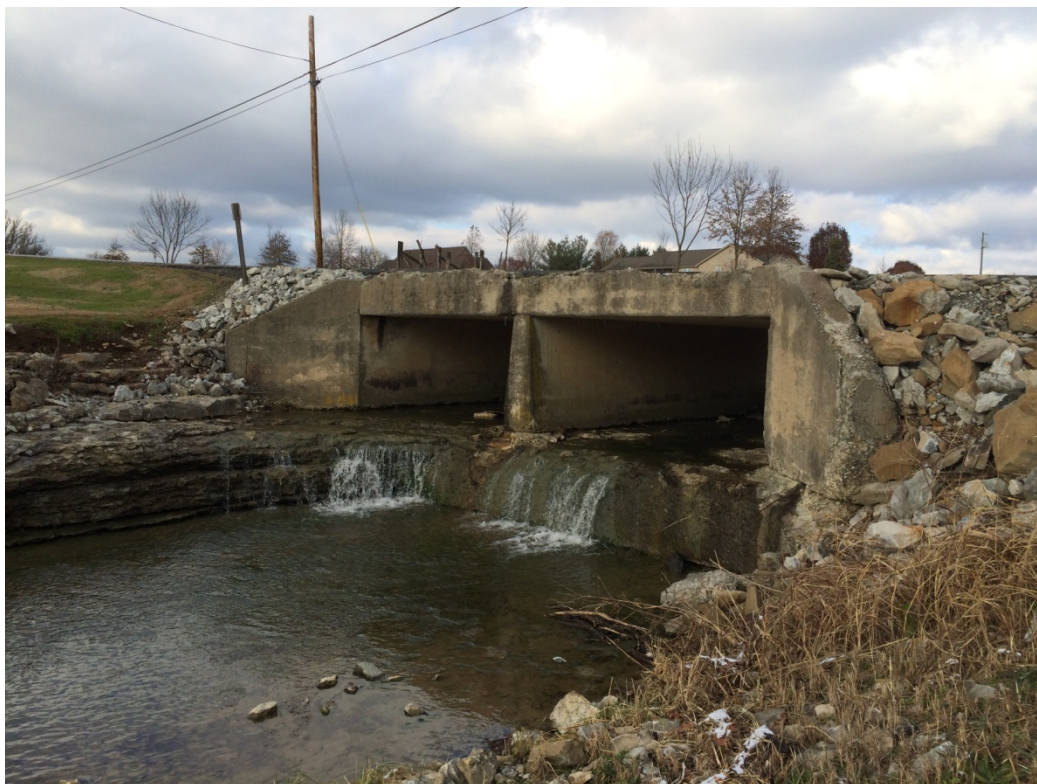
Outlet of existing culvert – rock scour of thin layers.
